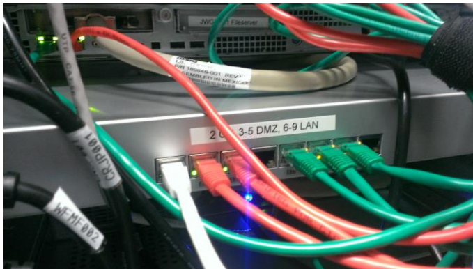
Firewalling co-located servers with RouterOS
